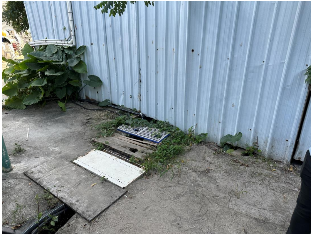
Photo 1: Hoarding without concrete footing
